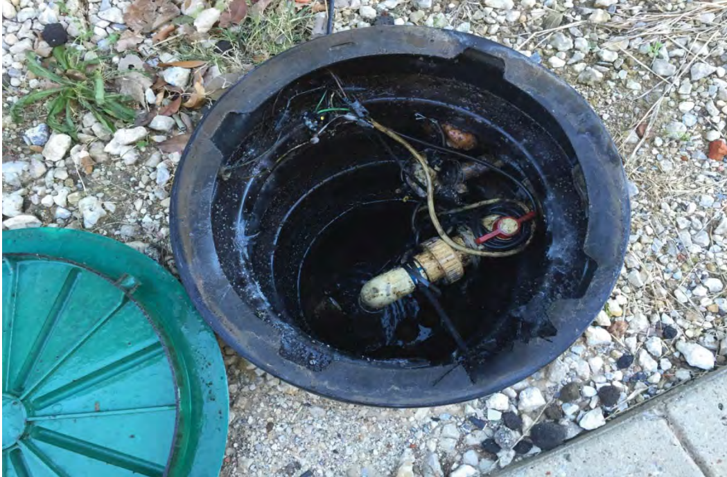
Photo P1: Sanitary Pump and Septic Tank
