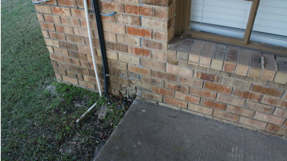
Photo S12. Cracking in Brick at Opposite Corner
