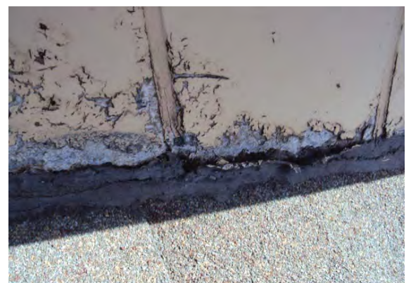
Photo A8. Deteriorating Sheathing
