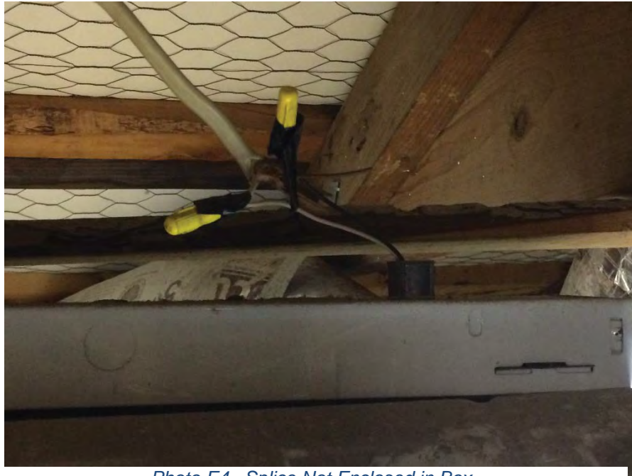
Photo E4. Splice Not Enclosed in Box
