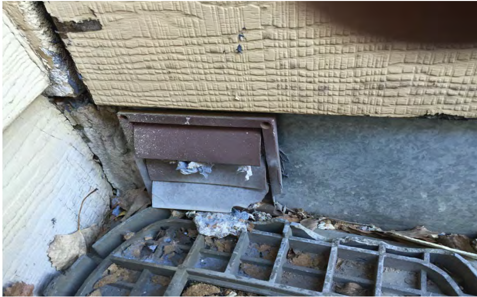
Photo M1. Clogged Dryer Exhaust Backdraft Damper
