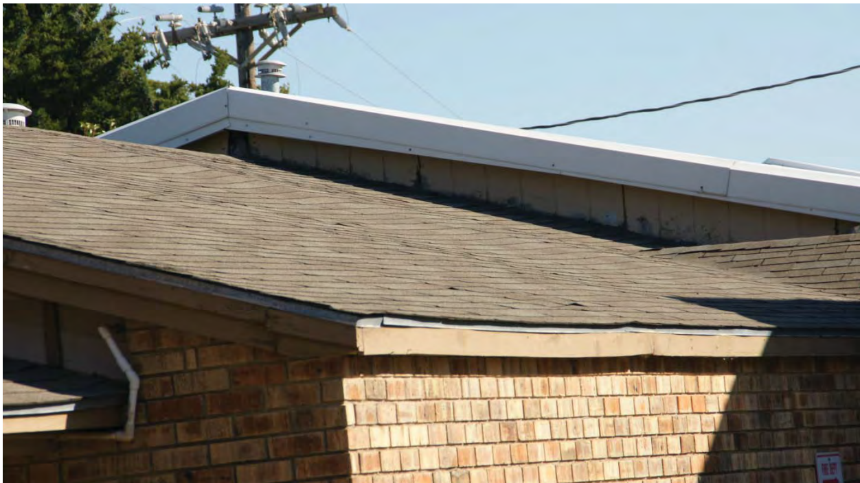
Photo S1. Ripples in Roof Over Original Construction (1960's) Module
