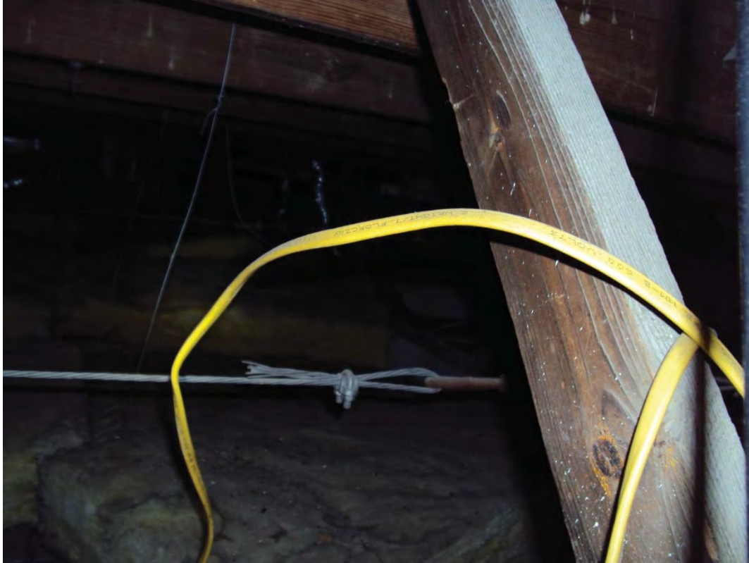
Photo S5. Cable Spanning Across Attic at East End of Attic
