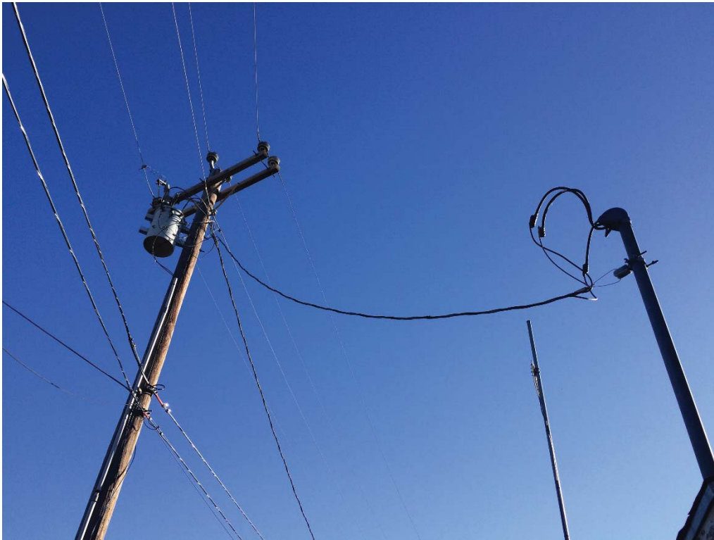
Photo E1. Overhead Service
