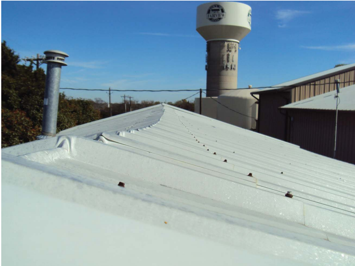
Photo A9. Roof Creep, Fatigue, Failure
