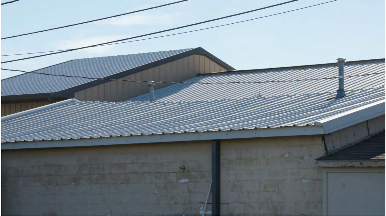
Photo S3. Sagging Roof
