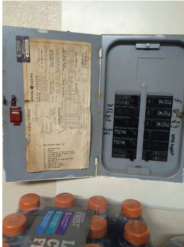
Photo E2. Sub-Panel Blocked by Stored Items
