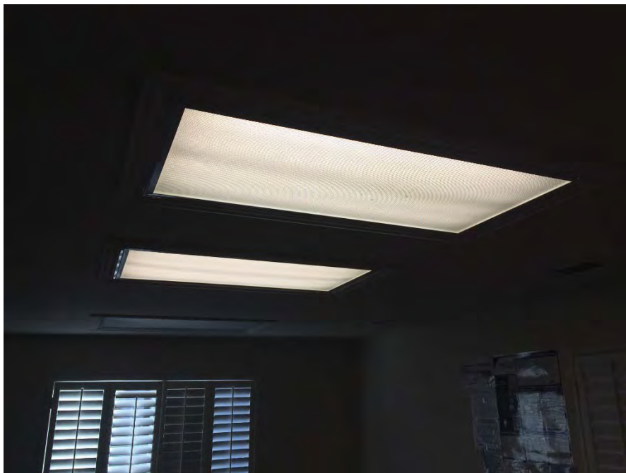
Photo E8. Typical Fluorescent Fixtures
