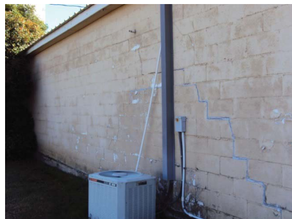
Photo A11. Cracks at Exterior Facade
