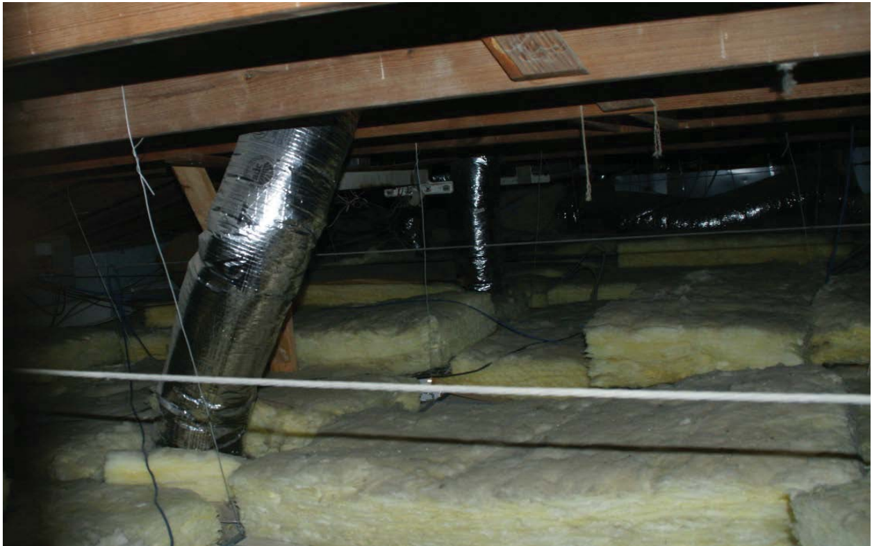
Photo S4. East End of Attic Space Over 1980's Addition. Notice Cable Tie In Foreground
