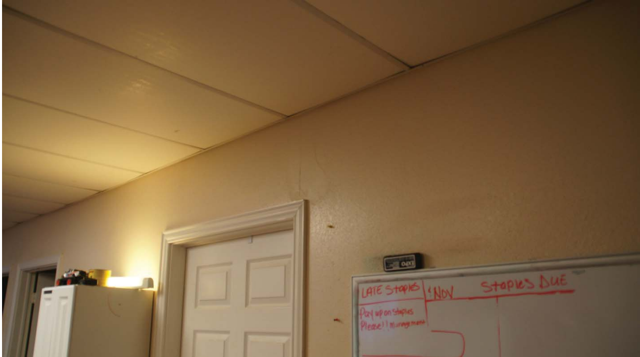
Photo S14. Cracking Above Doors on the Interior
