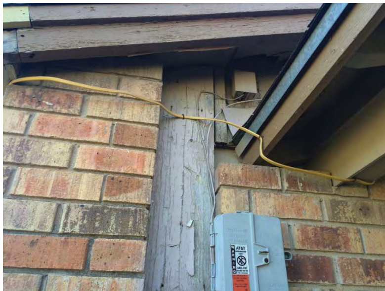
Photo E3. Improper Use of Type NM Cable
