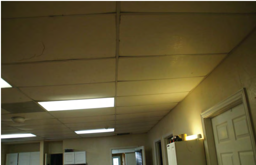
Photo S10. Suspended Ceiling Hung from Sagging Rafters – 1980's Addition
