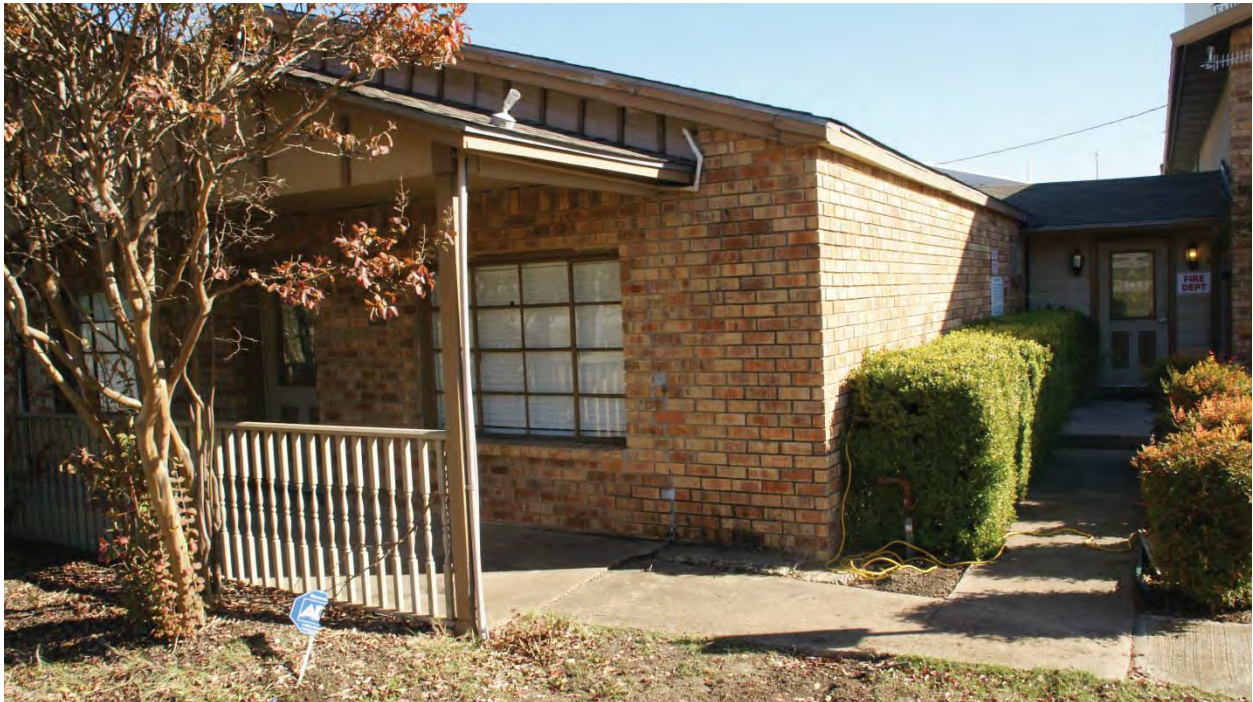
Photo S11. Cracking in Brick
