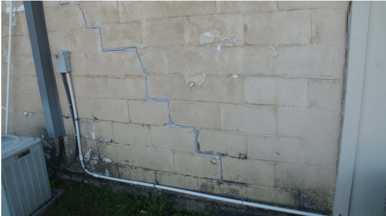
Photo S13. Cracking in CMU Due to a Combination of Foundation Movement and Lateral Thrust from Rafters
