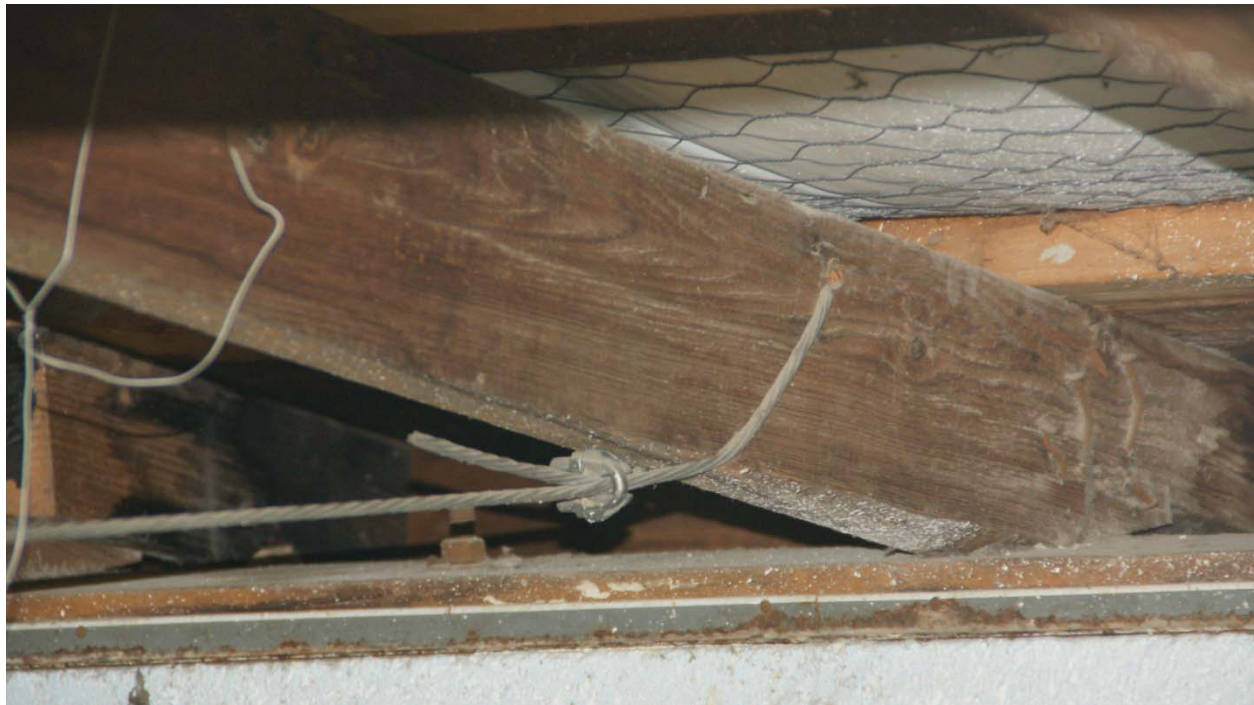
Photo S6. Cable Connection at Rafter
