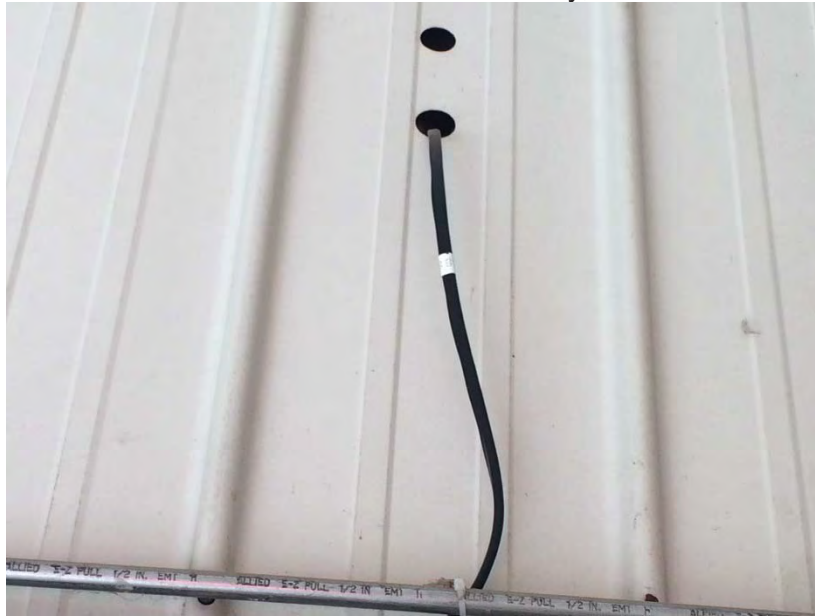
Photo E5. Cable Through Wall Panel Without Protective Bushing
