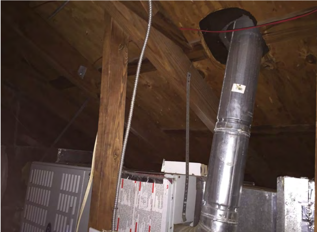
Photo S7. HVAC Equipment Suspended from Rafters
