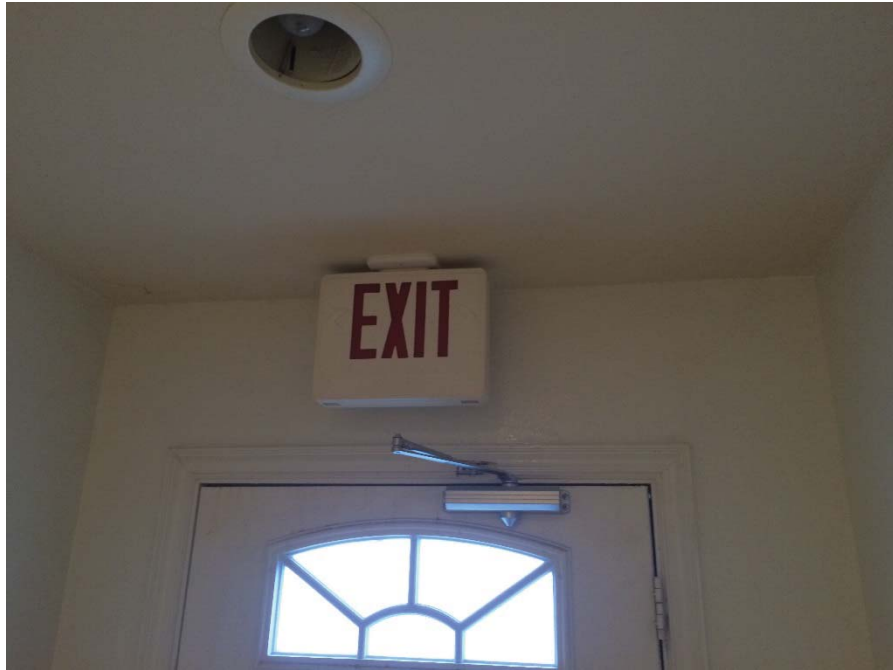
Photo E10. Exit Light Not Working
