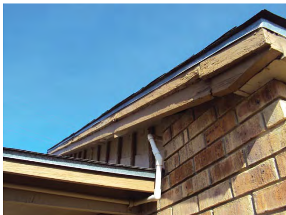
Photo A10. Wood Rake and Trim Rotting
