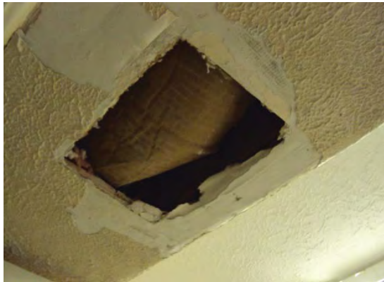
Photo A5. Roof Leak at Ceiling
